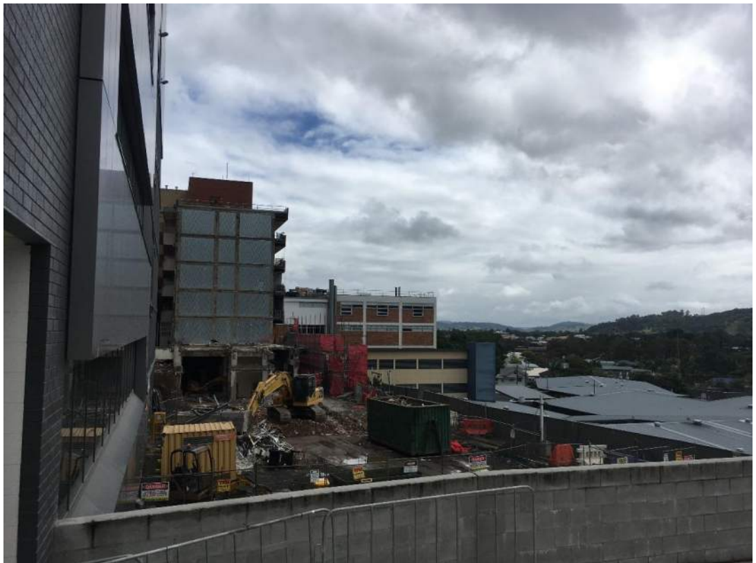
Figure 13: View of the construction site to the north of the Stage 3A and 3B1 buildings. The Stage 3B2 north tower is currently under construction (Source: JHG)
