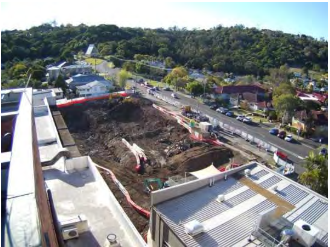
Figure 5: Excavation works at LBH site (Source: Supplied by City Plan Strategy & Development)
