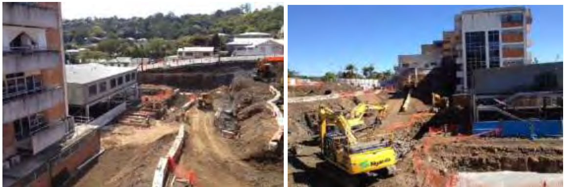
Figure 3: Excavation works at LBH site (Source: Supplied by City Plan Strategy & Development)
