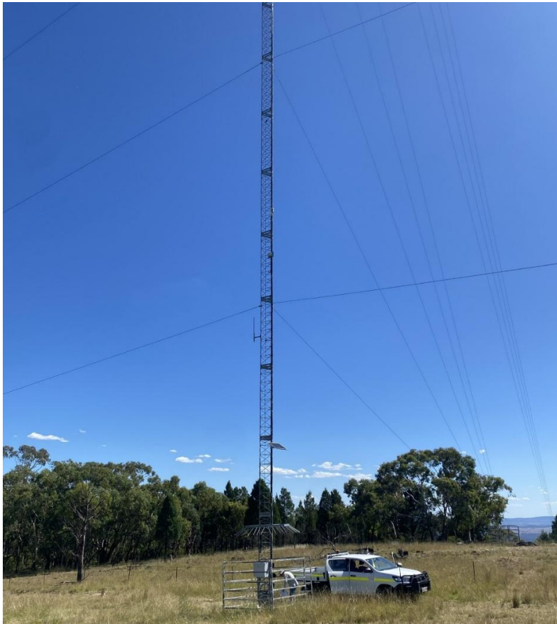
Figure 2-18: Temporary Met Masts
