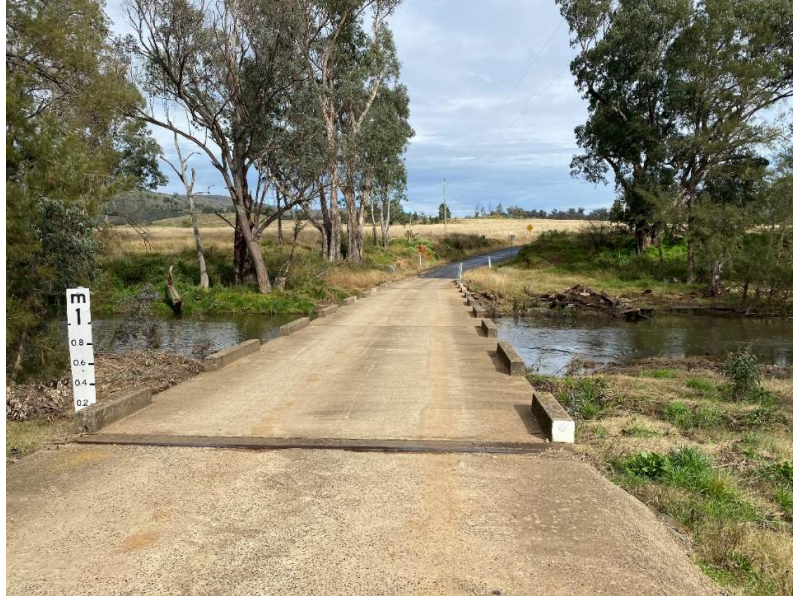
Figure 82 – Burrendong Dam Rd (CH 600) waterway bridge and insufficient curve in background
