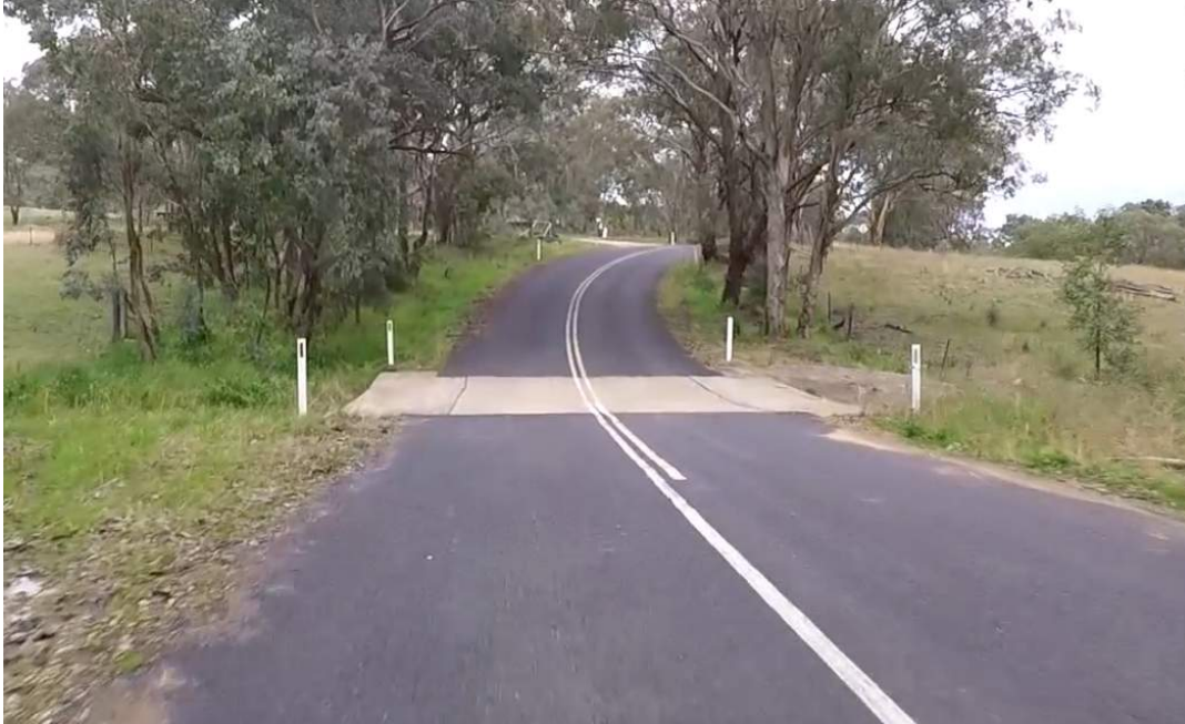
Figure 12 – Yarrabin Road CH 34,450 floodway and vertical curve.
