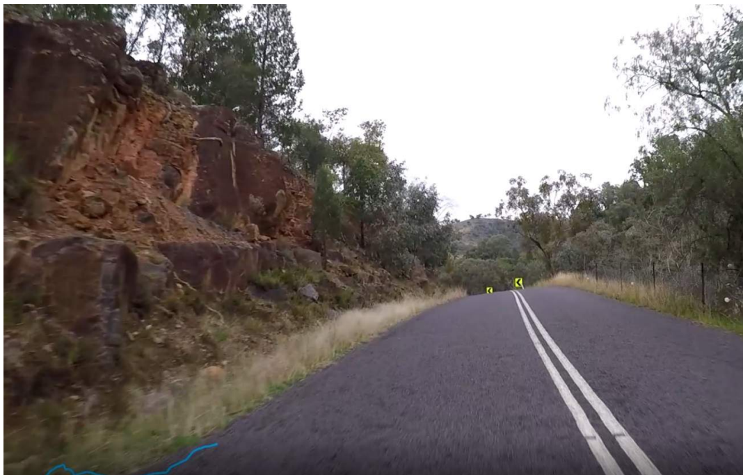
Figure 26 – Yarrabin Road CH 28,400. Rock wall at start of the bend, and drop off on right side of photo.
