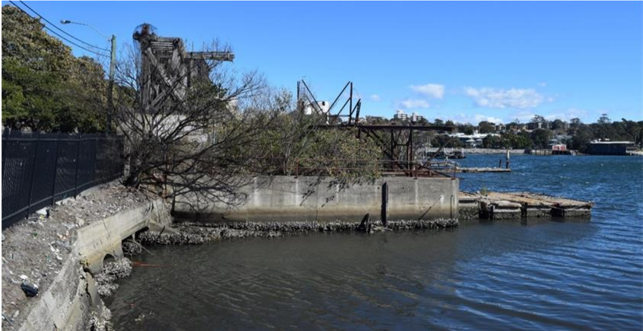
Figure 11: Eastern side of the former coal loader and viewed from the existing fish market.
