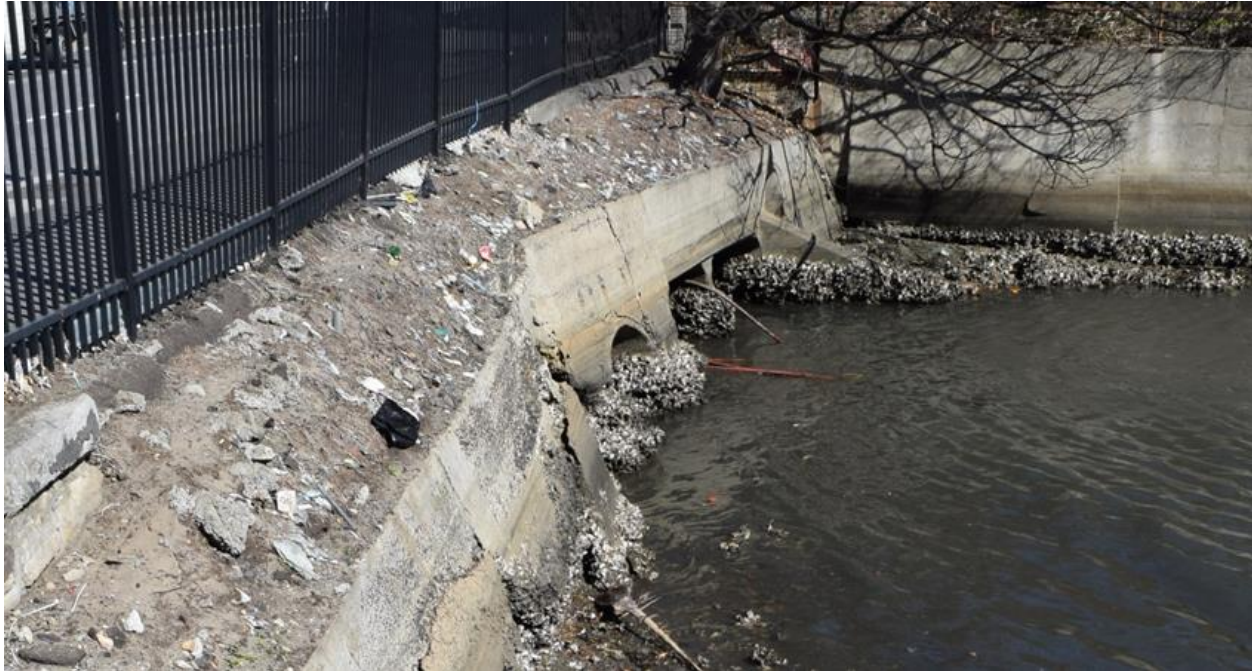
Figure 10: Stormwater outlets 17A-F and seawall located within the south eastern corner of the subject site.
