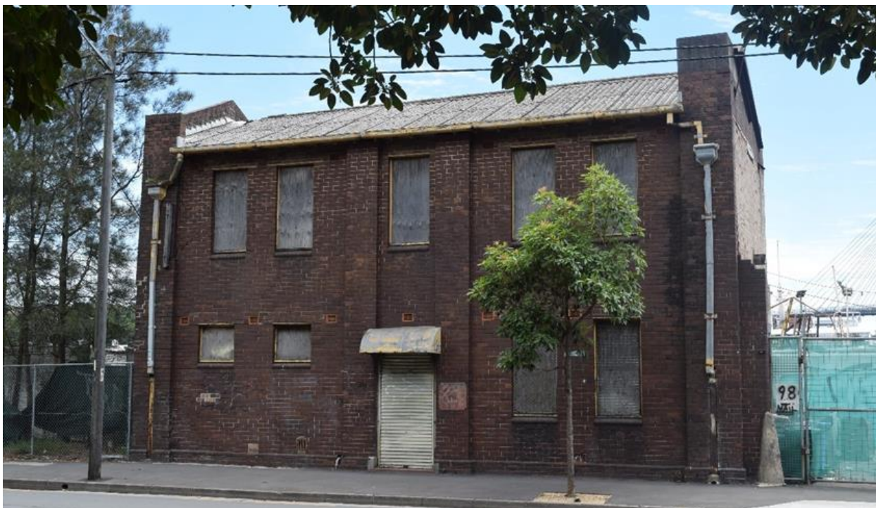
Figure 17: The southern façade of the former office/ weighbridge building, which is prominently visible from within Bridge Road.
