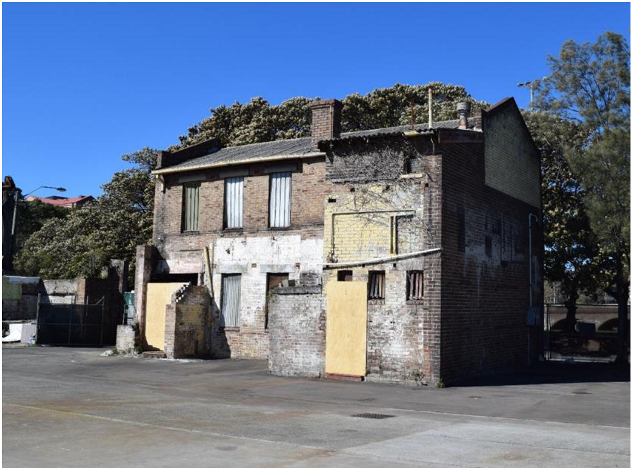
Figure 15: The northern and western facades of the former office/ weighbridge building. Note the structure has been boarded up.
