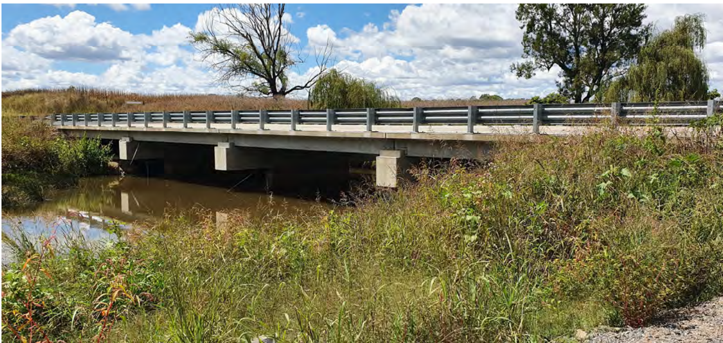
Plate 1-2. Recently completed bridge over the Macintyre River that was found to provide roost habitat for the Eastern Bent-wing Bat ( Miniopterus orianae oceanensis ).
