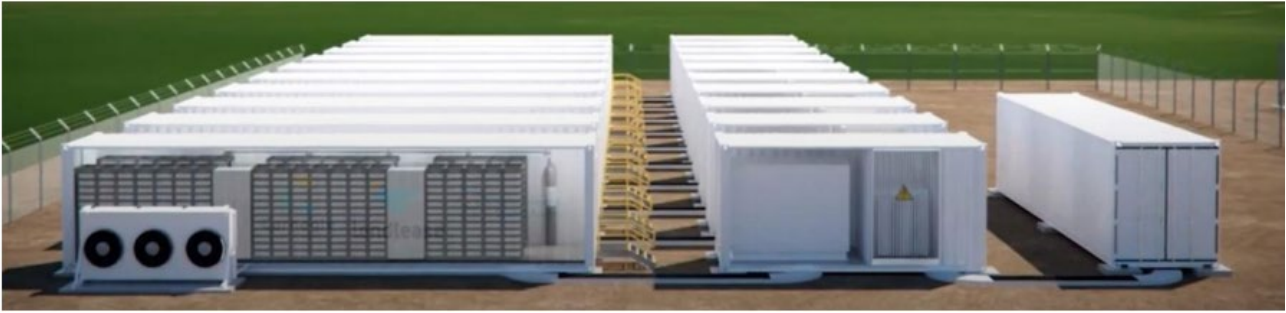
Photograph 2.2 Example of containerised batteries
