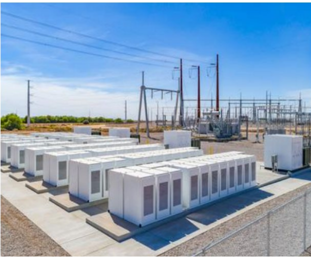
Photograph 2.3 Example of a modular battery solution
