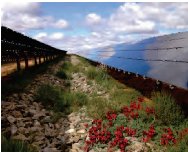
53 MW solar farm Broken Hill. Photo AGL
