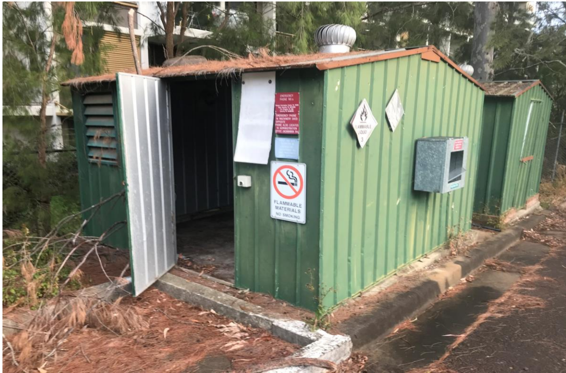
Photograph: 13 Eastern chemical store metal shed, with Flammable Goods signage, with adjacent possible bunded area
