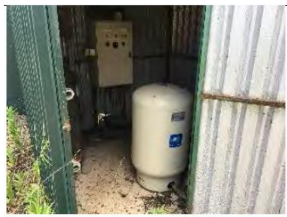
Photo 23 – Electric pump shed.
