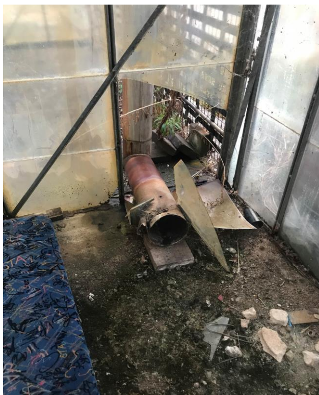
Photograph: 30 Pipes inside greenhouse
