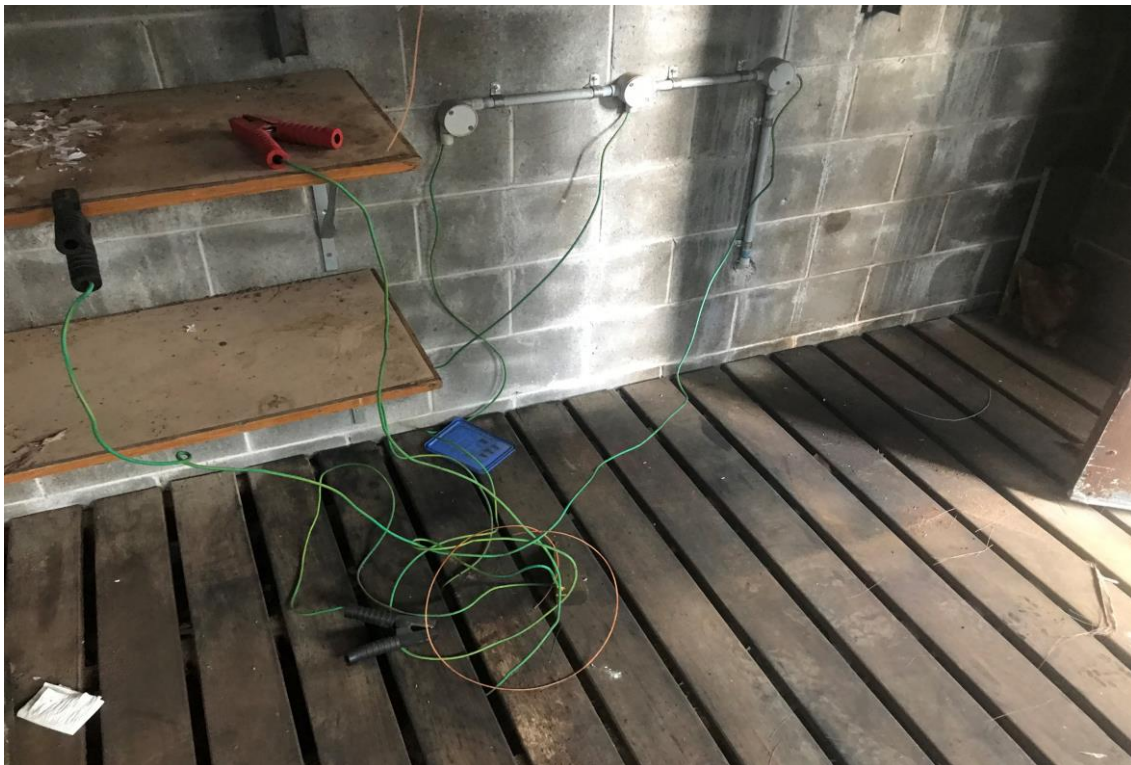
Photograph: 8 Besser Block Flammable Goods Store - indicators of battery storage and use and dark staining on floor boards
