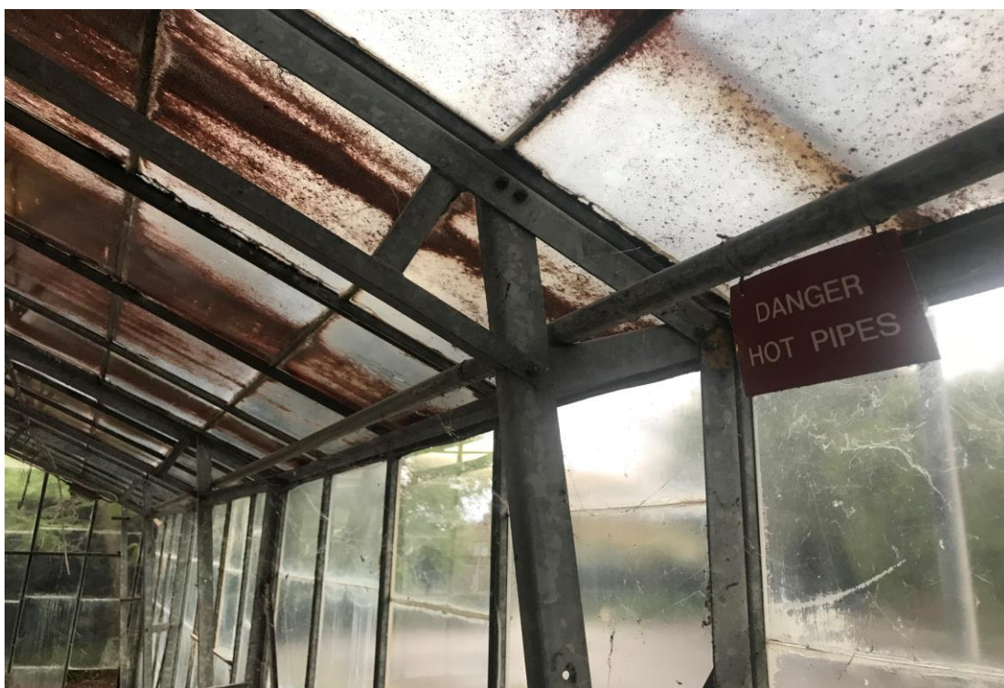
Photograph: 29 Pipes inside greenhouse
