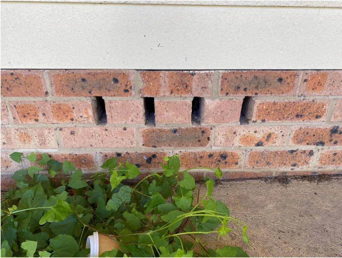
Figure 8: Ventilation holes in brick foundation walls of Block M which potentially allow microbat access to underfloor areas
