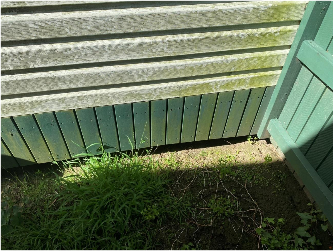
Figure 6: Gaps between boards covering underfloor openings and ground level, Block N
