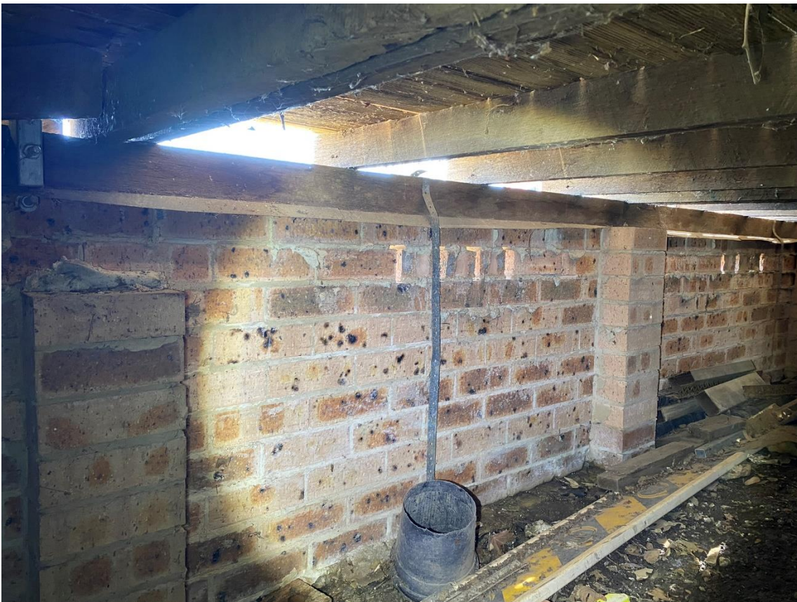
Figure 7: Gaps between floor and brick foundation wall, Block M
