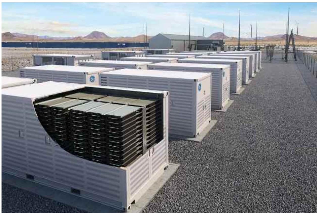
Figure 3-4: Typical BESS Arrangement
