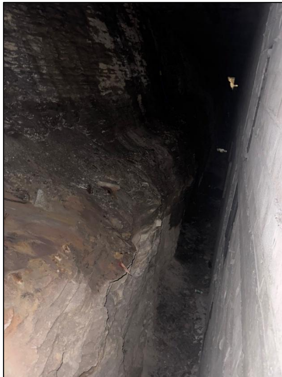
Plate 1: View looking north-west inside the air plenum of the neighbouring basement to the south-east
