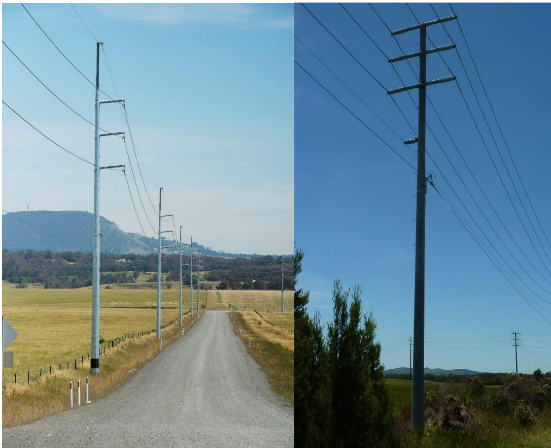
Figure 3 - Typical overhead 66 kV transmission lines
