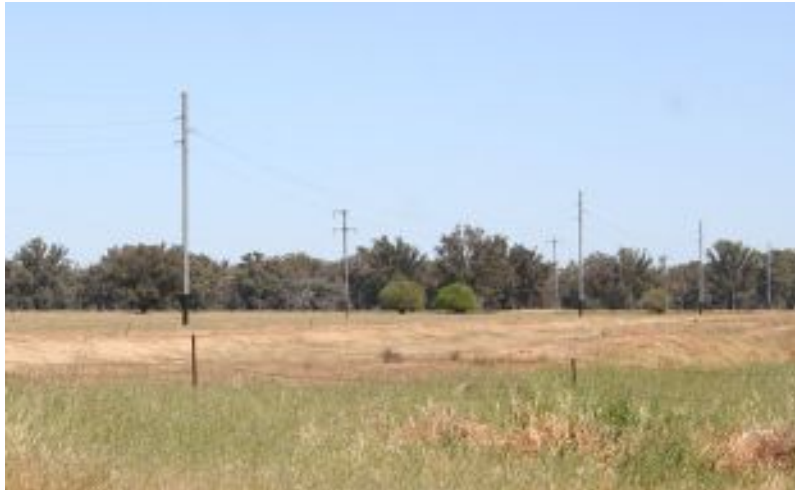
Figure 3.9 66kV transmission line recently installed in the vicinity (in foreground)
