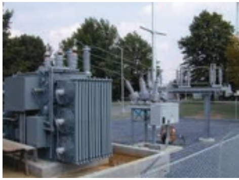
Figure 3.7 Typical fenced transformer station showing transformer and switchgear (photo: Vast Solar)
