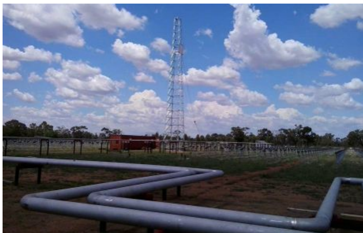
Figure 3.4 Thermal piping at Jemalong pilot plant before being insulated (photo: Vast Solar)
