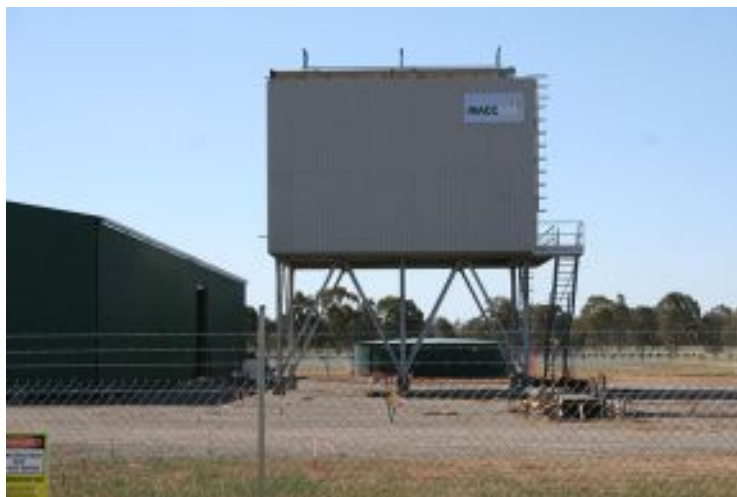
Figure 3.6 Air-cooled condenser at Jemalong pilot plant
