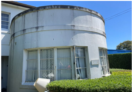
LS4: 255 Maroubra Road Exterior Metal windowsill.
