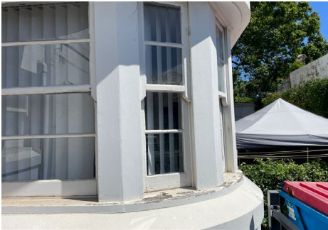
LS5: 255 Maroubra Road Exterior Wooden windowsill.
