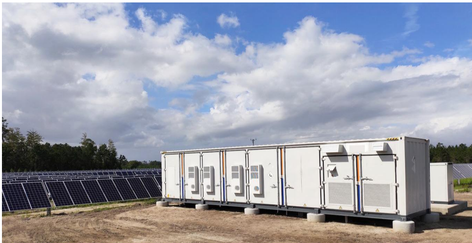
FIGURE 8 CLOSE UP EXAMPLE OF DISTRIBUTED BATTERY UNIT WITH INVERTER ADJACENT TO SOLAR PANELS (SOURCE: HTTPS://EN.SUNGROWPOWER.COM/NEWSDETAIL/2127 )
