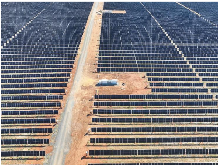
FIGURE 3 MARYVALE SOLAR FARM – BATTERIES INSTALLED
