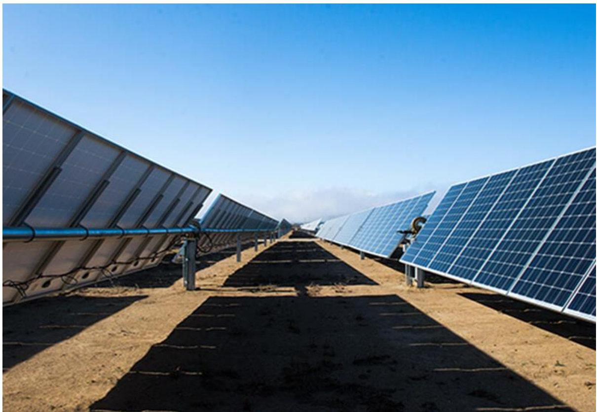
FIGURE 2 EXAMPLE OF TRACKING SOLAR PV PANELS
