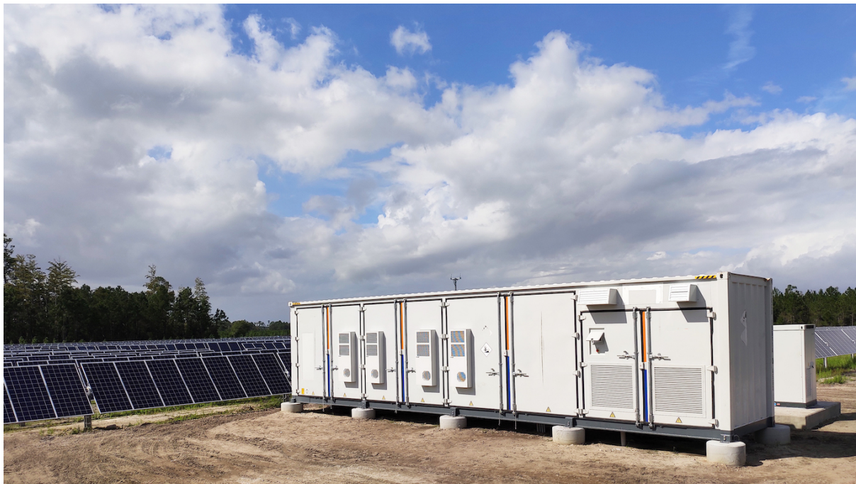
FIGURE 7 CLOSE UP EXAMPLE OF DISTRIBUTED BATTERY UNIT WITH INVERTER ADJACENT TO SOLAR PANELS (SOURCE: HTTPS://EN.SUNGROWPOWER.COM/NEWSDETAIL/2127 )
