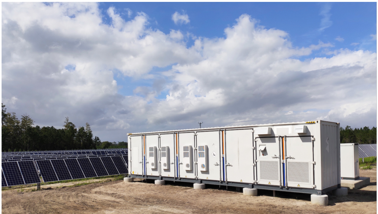
FIGURE 9 CLOSE UP EXAMPLE OF DISTRIBUTED BATTERY UNIT WITH INVERTER ADJACENT TO SOLAR PANELS (SOURCE: HTTPS://EN.SUNGROWPOWER.COM/NEWSDETAIL/2127 )
