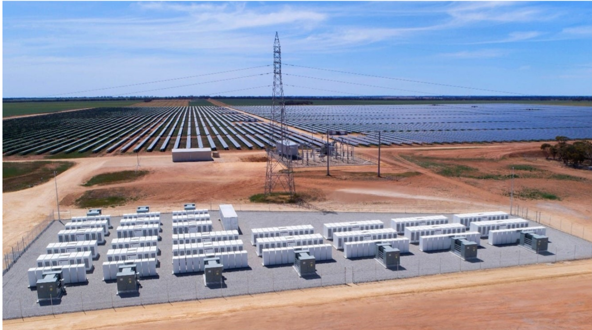
FIGURE 4 ILLUSTRATION OF A TYPE OF BESS COUPLED WITH A SOLAR FARM (SOURCE: WWW.ENERGYAUSTRALIA.COM.AU/ABOUT-US/ENERGY-GENERATION/GANNAWARRA-BATTERY-STORAGE )
