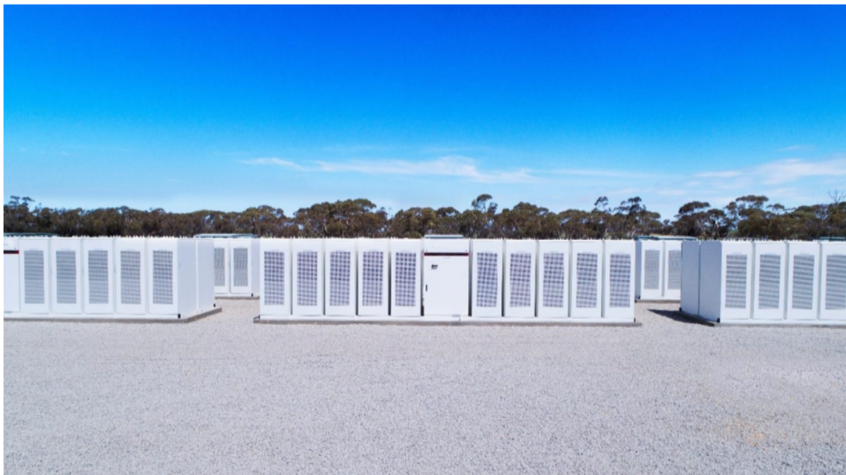
FIGURE 5 ILLUSTRATION OF CLOSE UP OF INDICATIVE BATTERY UNITS FOR ONE TYPE OF BESS (SOURCE: WWW.ENERGYAUSTRALIA.COM.AU/ABOUT-US/ENERGY-GENERATION/GANNAWARRA-BATTERY-STORAGE )
