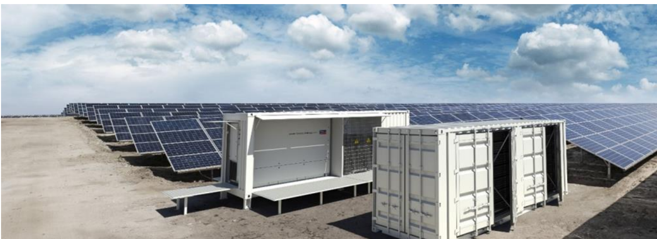
Figure 3-4: Example Inverter Station
