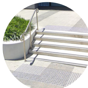
3 Fading concrete steps
