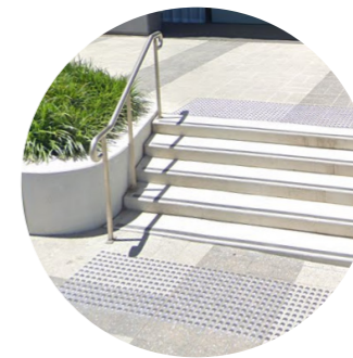
3 Fading concrete steps
