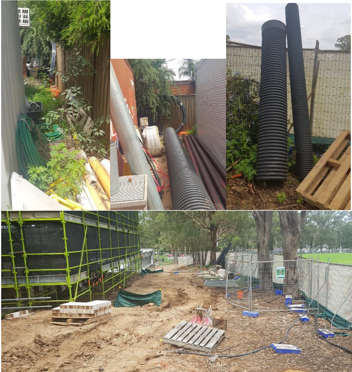
Photo 8: Series showing poor housekeeping
