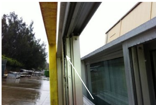
Photograph 07: Asbestos containing mastic in the groove of the window where the glass pane is inserted
