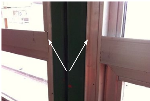
Photograph 06: Position where asbestos containing mastic is used to seal the join between the steel frame of the demountable and the aluminium frame of the windows / panels
