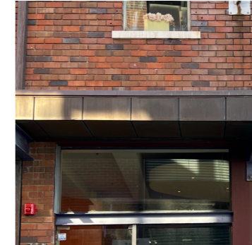
RSC - Copper awning
