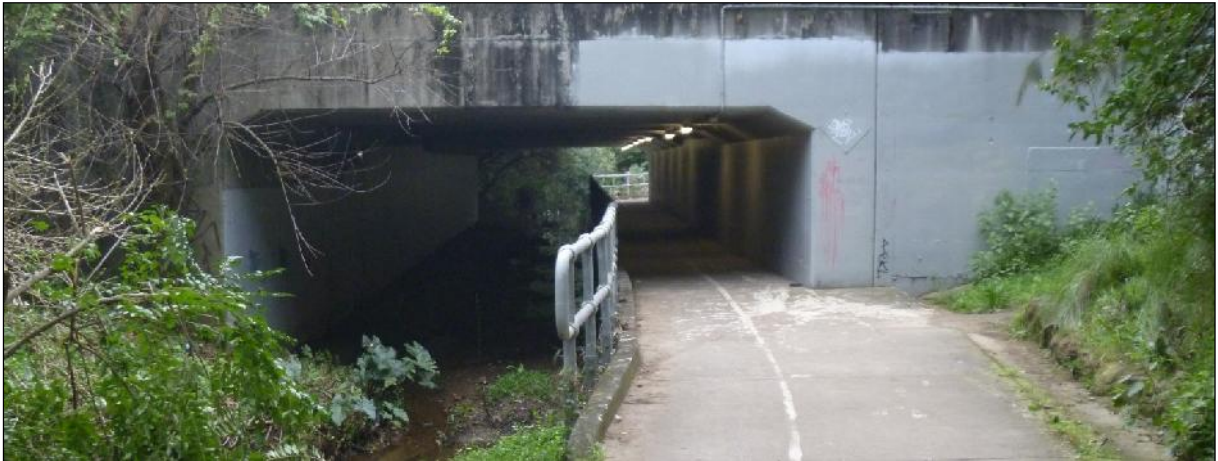
Figure 4: Epping Road Culvert for Shrimptons Creek, facing south. Note low sandstone outcrop (Feature "G") at right hand side of path.
