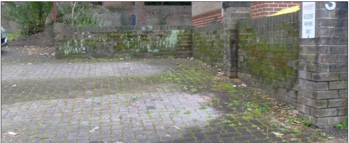
Figure 7: Moss growth on pavers and walls; 3 Wilcannia Way
