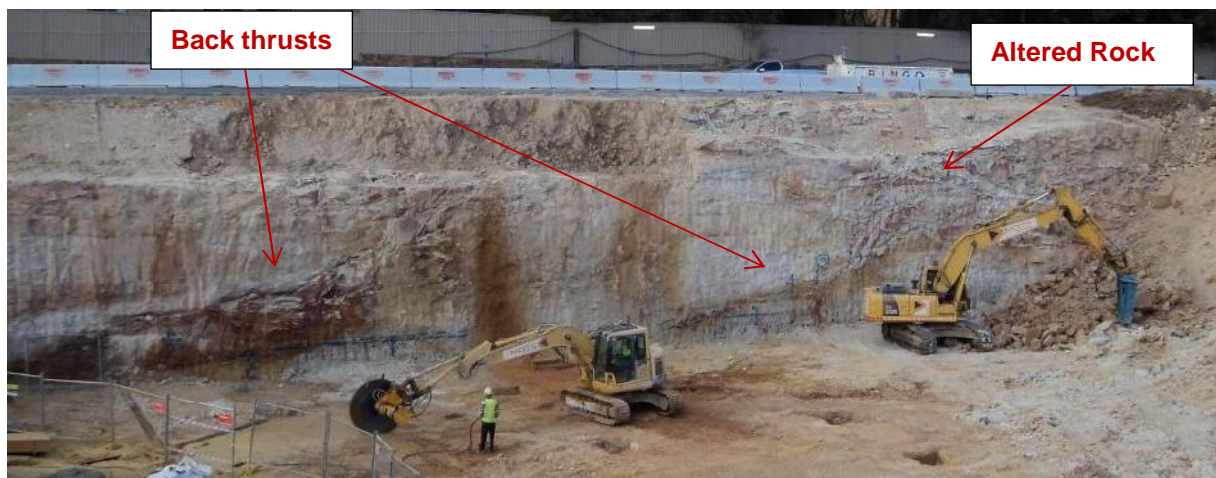
Figure 13: Back thrusts in an excavation wall at a nearby site
