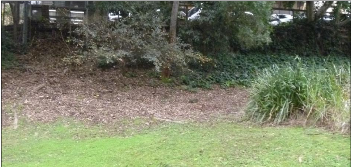
Figure 2: Mulched batter slope and crib wall at rear boundary between 2-4 and 6 Lyon Park Road
