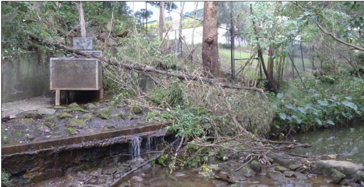
Figure 3: Stormwater outlet at Shrimptons Creek, with concrete sidewalls and sandstone boulder headwall, as viewed from north-western bank.
