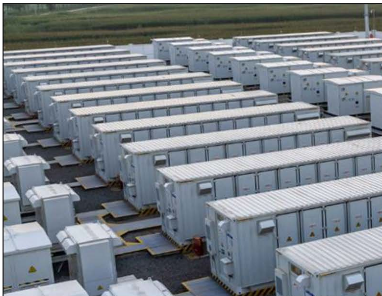
A generic view of a Battery Energy Storage System.
