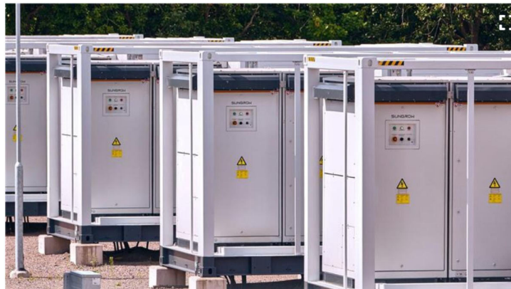
Batteries similar to these are proposed at a $135 million facility at Corowa to store solar energy.
