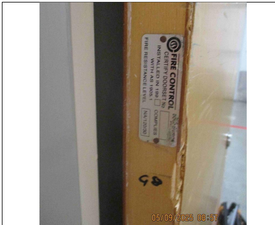
Photo 13 Corridor at Waste Bin Rooms. Fire Door G8. Tag dated "199_" year of manufacture.
