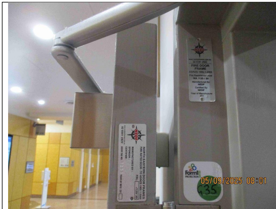
Photo 5 Foyer area near lifts, Fire Door G35. Tag dated “2015” year of manufacture.
