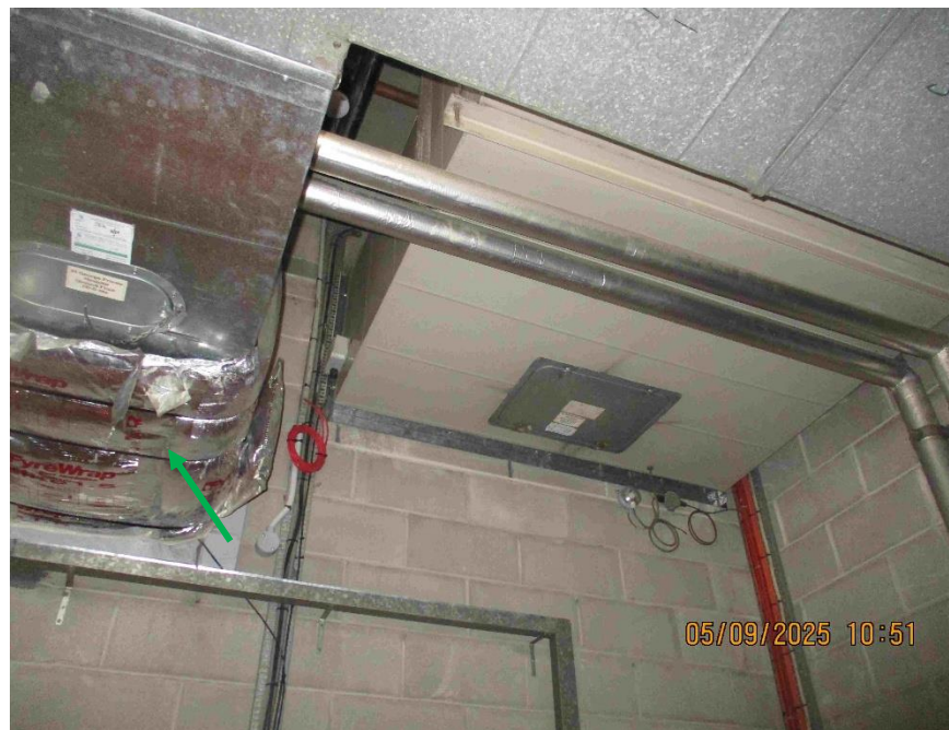
Photo 16 Plant Room, Air Handling Unit, G1, G2. FyreWrap duct insulation. Synthetic Mineral Fibre (SMF).
