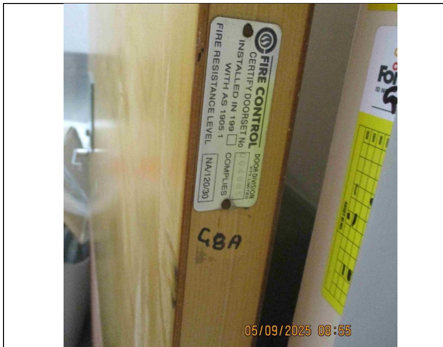
Photo 15 Clean Bin Store. Fire Door G8A. Tag dated "199_" year of manufacture.
