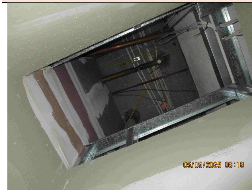
Photo 8 Fire Hose Reel cupboard at corridor to Discharge Lounge. Walls, plasterboard. Ceiling, concrete slab floor above.
