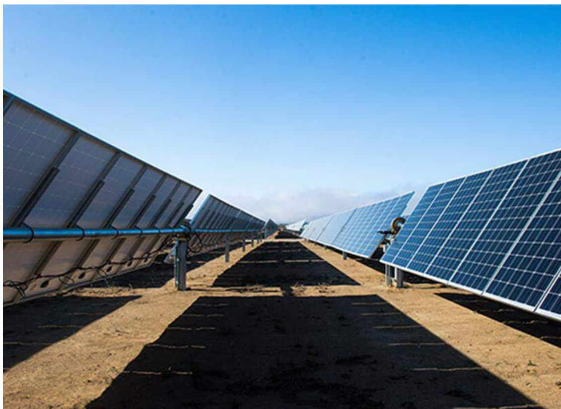
Figure 3-5: Example of Tracking Solar PV panels
