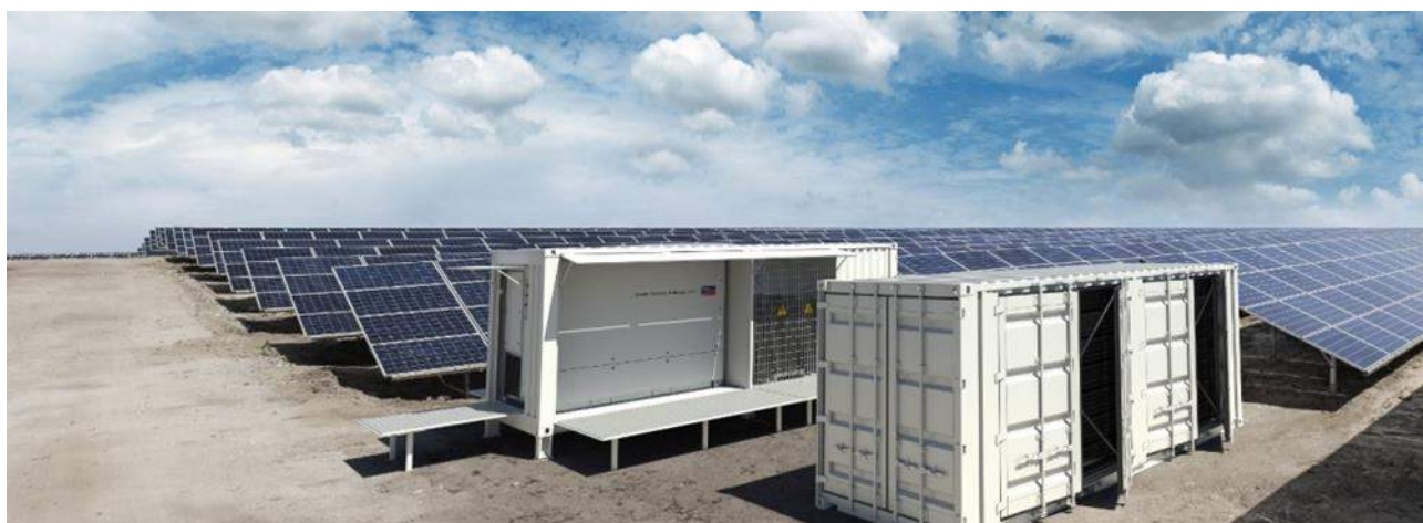
Figure 3-7: Example inverter station
