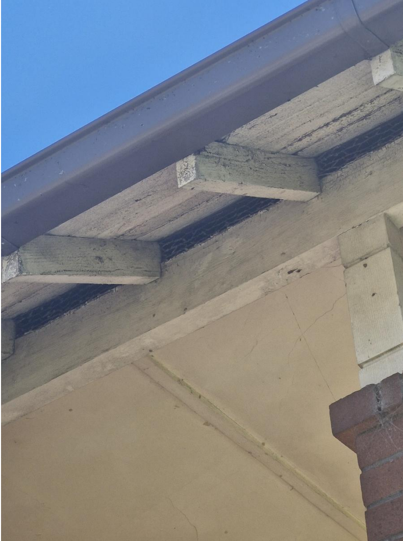
Photo 6 Open eaves with mesh barrier found on disused residential building within the study area
