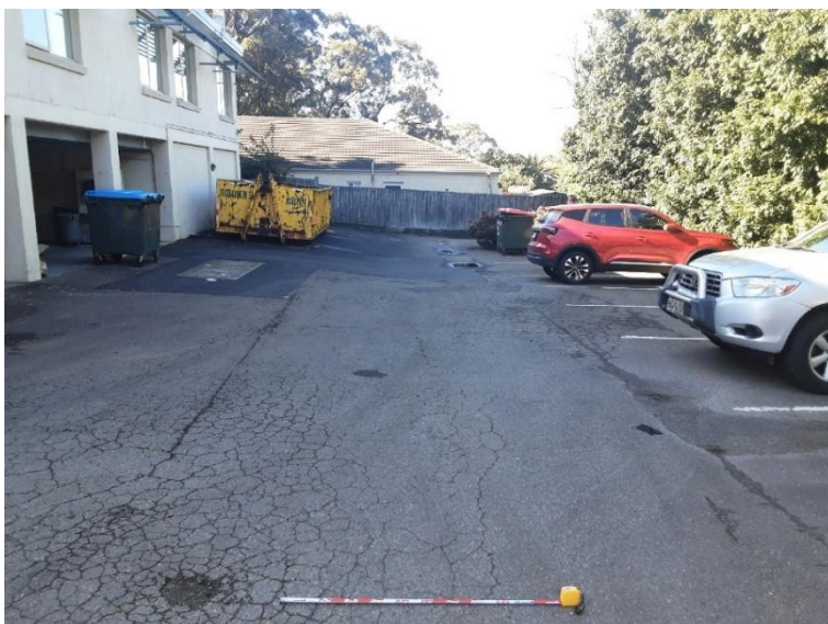
Photo 12 No GSV (0%) in the southern portion of 134 Beecroft Road, facing south-east (scale rod: 1 metre)
