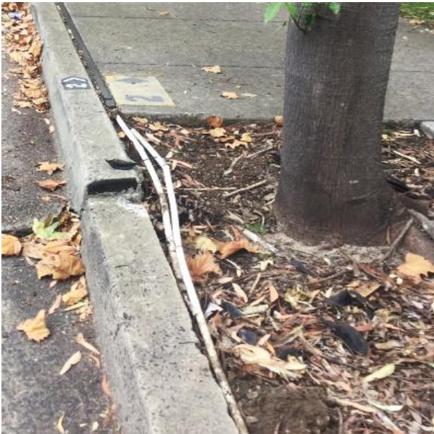
Figure 5: cable housed in white conduit
