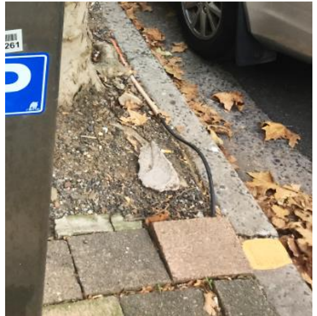
Figure 6: black cable housed in orange conduit
