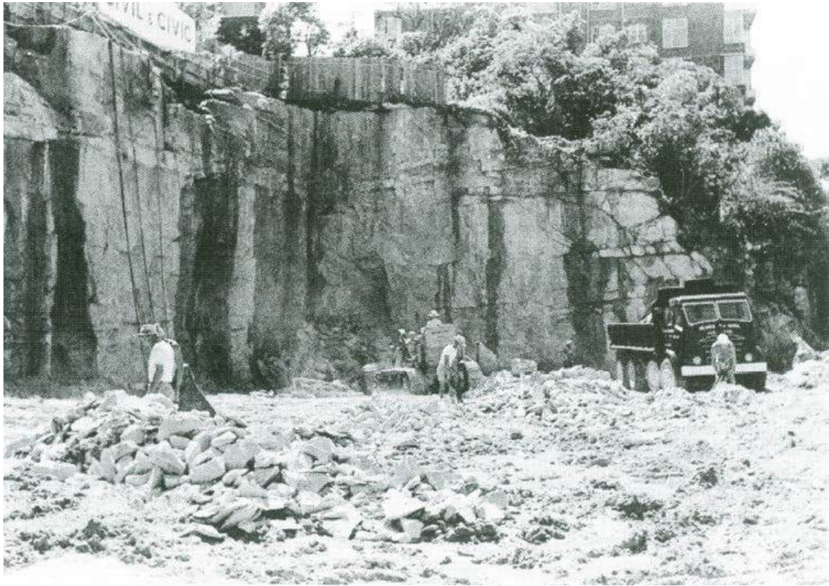
Figure 2.10: Excavation of sandstone in the Old Junior School yard area in 1962 to prepare for new buildings fronting Jeffreys Street and Kirribilli Avenue. Strong 1997:23.
