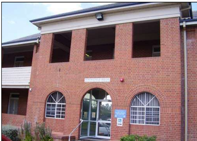
Figure 3.106 Aluminium framed windows and doors have also been added to the central bay, ground floor openings.
