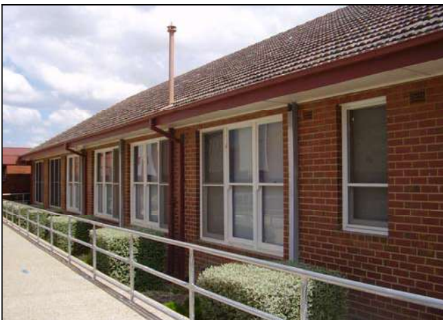
Figure 3.195 The 1950s, western portion of the building retains timber framed windows. Note the landscaping, path and railing recently added to the front of the building.
