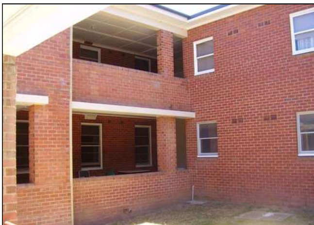
Figure 3.128 The Gerathy Wing has been constructed to the north western corner of the building.
