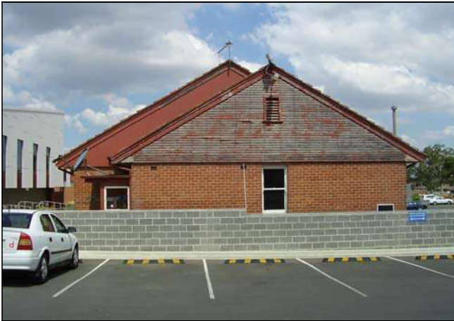
Figure 3.193 The western façade of the building which retains the original double gable timber boarding and vent and sheeted finish to the gable ends.
