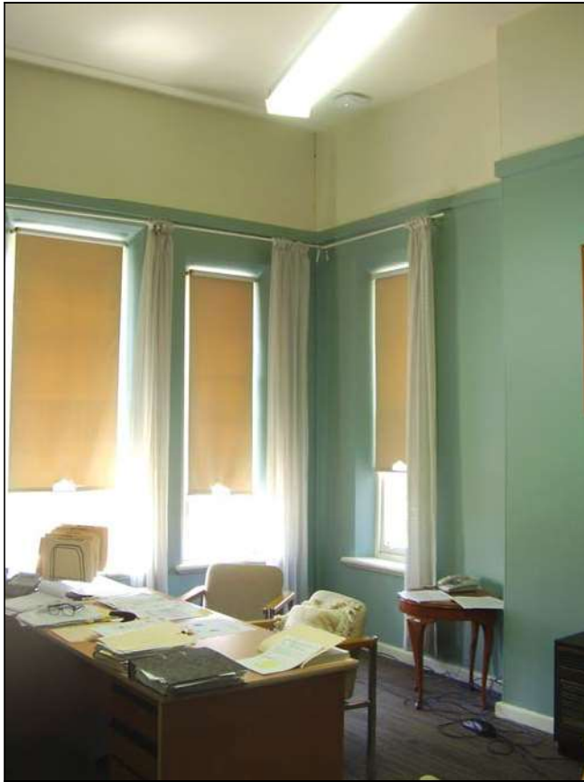
Figure 3.94 An office located on the first floor of the western pavilion. The space has generally been modified, however, also retains early features including fireplace breast (fireplace removed and infilled) timber joinery, high ceiling, windows and sills.
