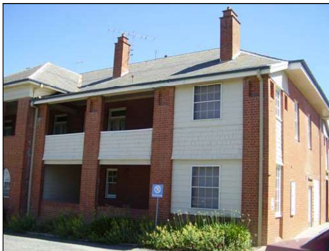
Figure 3.108 The north western corner and facades of the building. Note the lightweight infill to the end bays.
