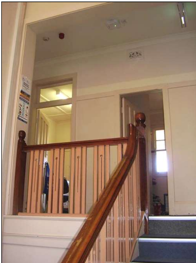
Figure 3.120 The first floor landing. The upper level also retains the double loaded layout and details including timber joinery.
