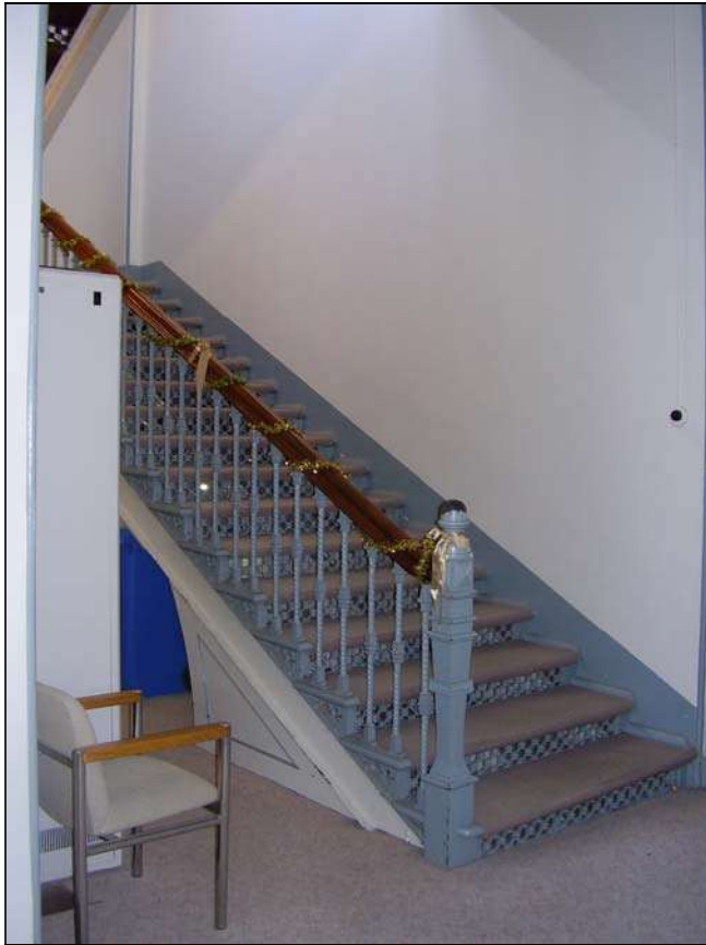
Figure 3.90 Each of three two storey pavilions retains a cast iron stair. The treads have been carpeted, however, the iron balustrade and timber handrails are in intact.
