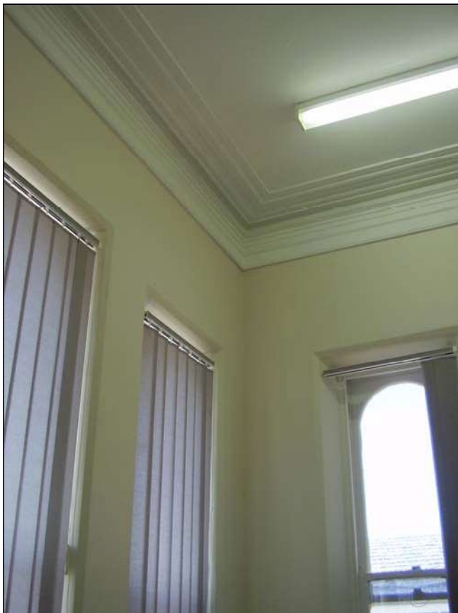
Figure 3.97 An office area in the western pavilion which also retains some profiled cornice.
