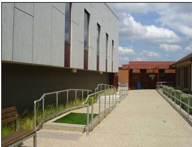
Figure 3.191 The paving and landscape elements, including rehab fixtures located to the south of the building.
