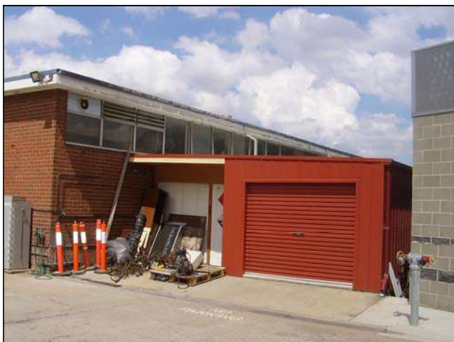
Figure 3.206 A skillion roofed shed/structure has been constructed to the southern facade of the building.
