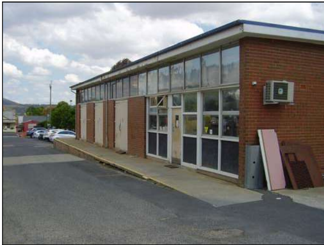
Figure 3.204 The northern façade of the building with has brick and both aluminium and steel framed glazed windows.
