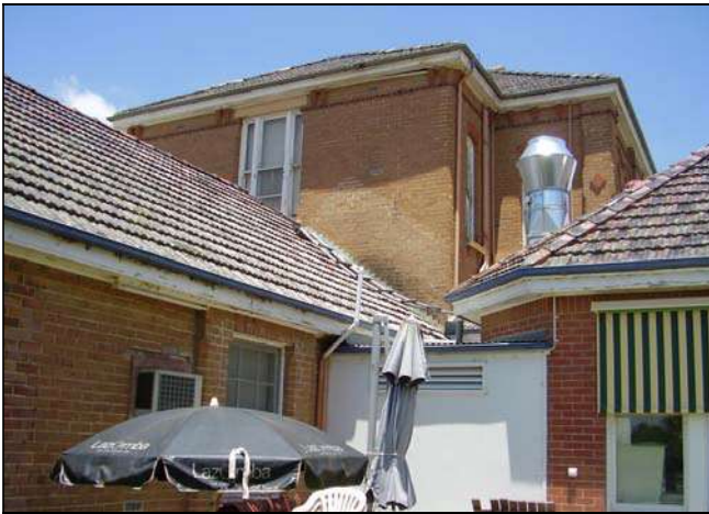
Figure 3.63 The northern façade of the two storey western pavilion also retains evidence of the original roof form over the original north western single storey wing.
