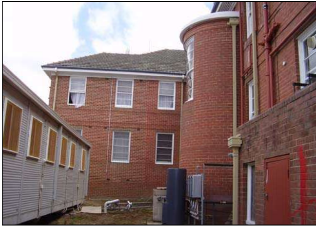
Figure 3.135 The brickwork at the south western section of the building indicates the extend of the 1950s addition. The southern façade also retains the curved bay with the main stair and a separate concrete and brick stair and arched opening accessing the laundry and service area in the building.
