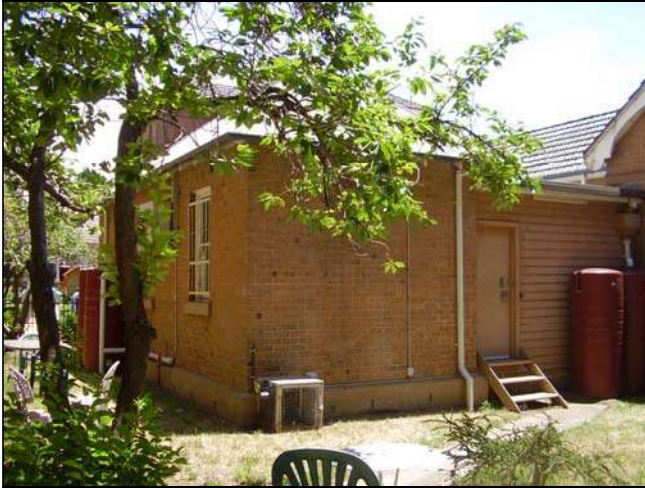
Figure 3.68 Additions dating from c. 1924 and 1960s at the western side of the original kitchen wing (now the Pharmacy).
