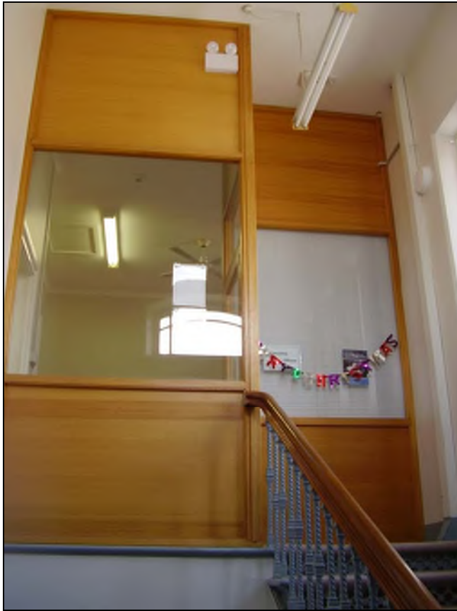
Figure 3.96 A partition has been added to the top of the western stair, however, the stair and void remains.
