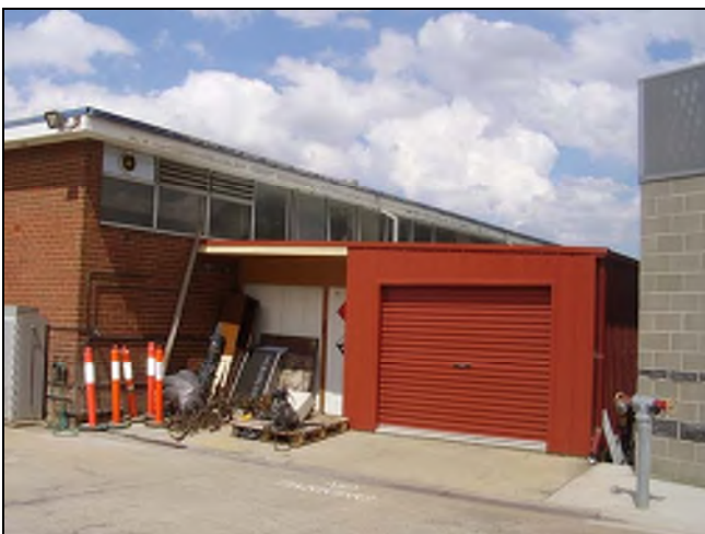
Figure 3.206 A skillion roofed shed/structure has been constructed to the southern facade of the building.
