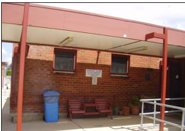
Figure 3.196 The eastern wing was added in the 1970s and accommodates Physio and Occupational Therapy. The entry also has a flat roofed canopy supported on simple steel posts.
