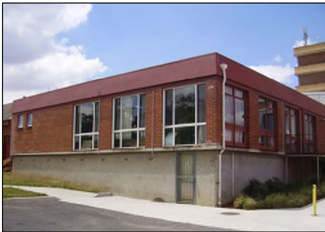
Figure 3.198 The eastern and southern façade of the 1970s addition to the building. A concrete ramp also extends along the north eastern façade.
