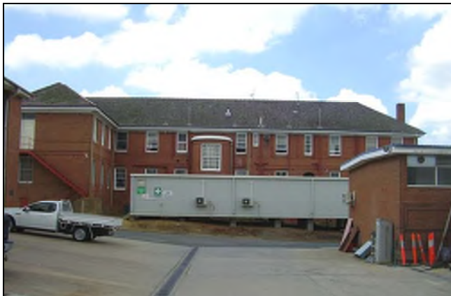
Figure 3.134 The “rear”, southern façade of the building faces the access road and service buildings in the mid section of the site. A demountable structure has also been added to the open area behind the building.
