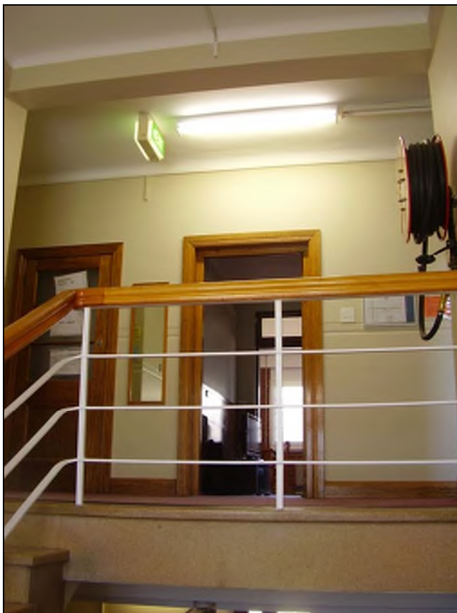
Figure 3.144 The first floor landing that retains the original steel balustrade with timber handrail and simple finishes.
