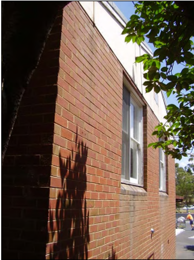
Figure 3.165 The south western façade of the southern wing which has a battened sheet finish to the gable end.
