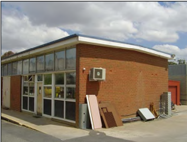
Figure 3.205 A concrete apron and sealed areas extends around the front and western side of the building.
