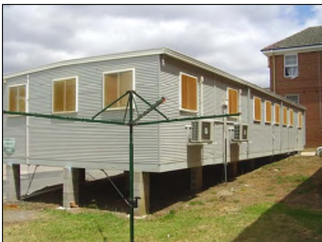
Figure 3.240 The north and eastern façades of the demountable which is mounted on concrete block piers.
