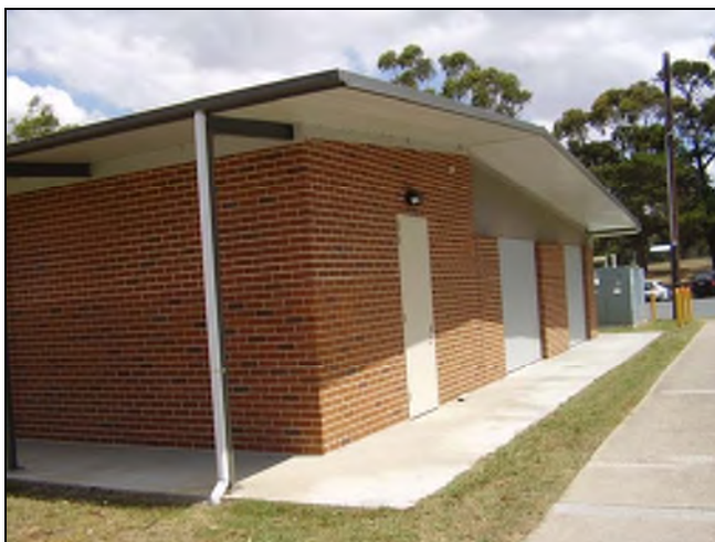
Figure 3.232 The Albert Street façade of the structure which has wide, extended eaves and concrete apron around the building.
