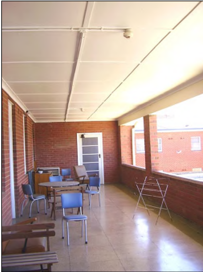
Figure 3.147 The first floor balcony which also has terrazzo floor finish, solid brick balustrade and batted ceiling.
