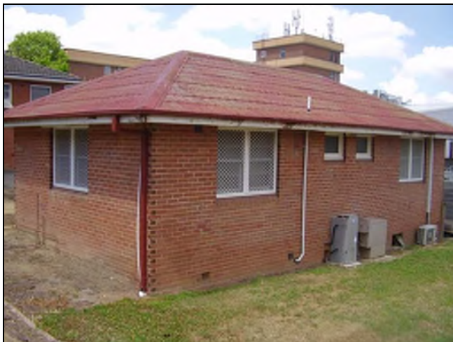
Figure 3.169 The western and southern facades of the building. Security screens have been added to the building with services.
