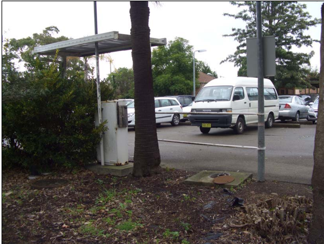
Photograph 1: Fuel Dispenser, Canopy and Remote Fill Point – facing southwest
