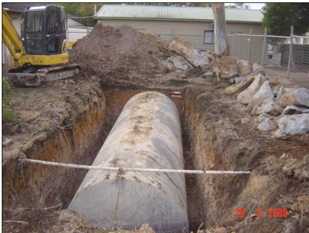
Photograph 4: Exposed UST – facing east
