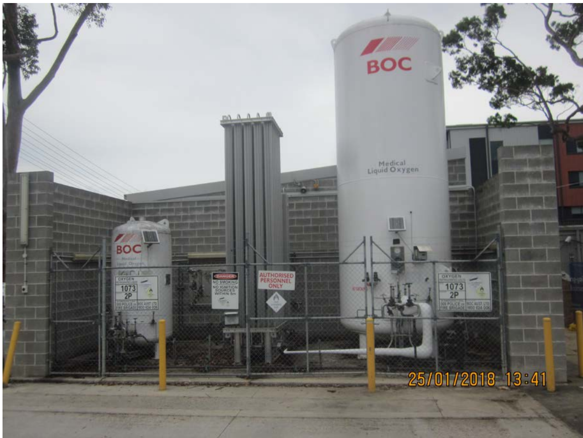
The existing bulk liquid oxygen tanks
