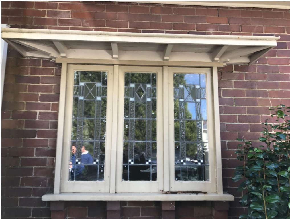
Figure 74: Detail of front window, glazing and hood. Note to the above right of the window, the building displays evidence of structural cracking which is expected to be caused by reactive clay soil under the foundations.
