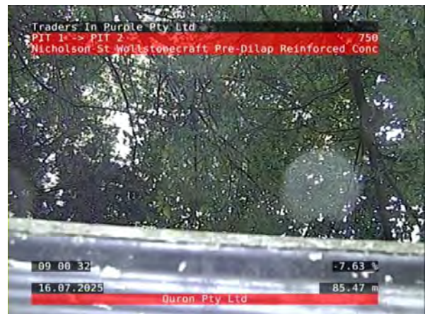
16, 00:14:40, 85.47 Obstruction, an object has been built into the structure, Obstruction: 5-20% from 10 o'clock to 2 o'clock, Finish # /
