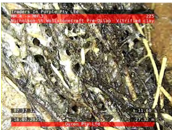
5, 00:05:39, 27.32 Fine roots--a relatively small number of flexible minor roots, at joint, Obstruction: <5% from 4 o'clock to 5 o'clock
