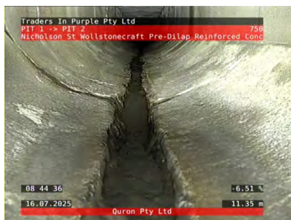
4, 00:03:15, 11.35 Other surface damage, SCOURING, Obstruction: <5%, Start #
