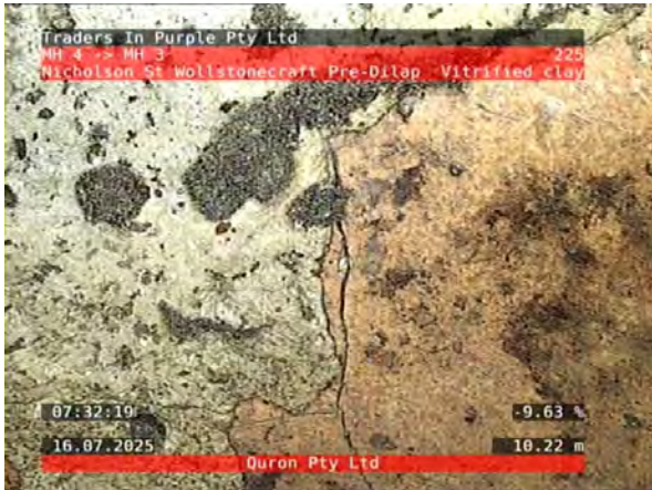
1, 00:01:47, 10.22 Longitudinal wall crack, at joint, width: 0.1mm at 1 o'clock
