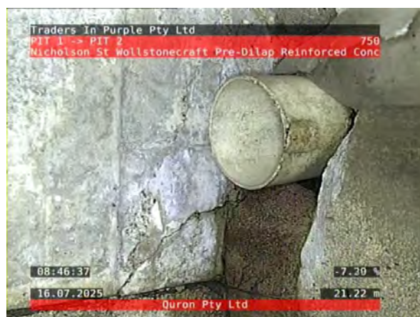
6, 00:04:52, 21.22 Connection, good workmanship, connection appears to be open, height: 100mm at 1 o'clock
