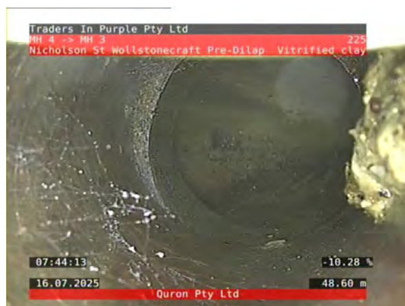
12, 00:10:30, 48.60 Junction open, good workmanship, height: 150mm at 3 o'clock
