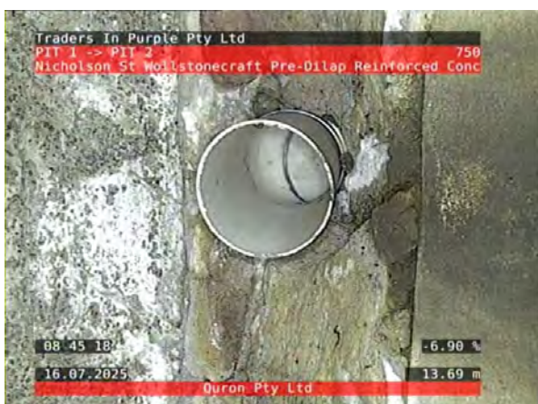
5, 00:03:42, 13.69 Intruding connection, magnitude of intrusion: <5% at 1 o'clock
