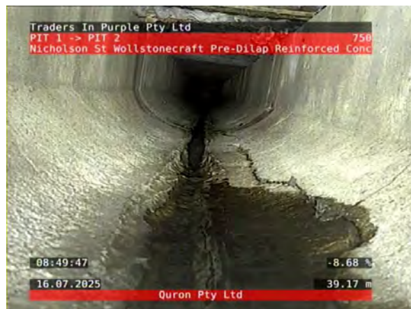
8, 00:07:37, 39.17 Longitudinal fracture, width: 2mm at 6 o'clock, Start #
