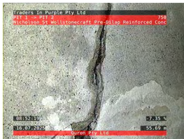
10, 00:09:42, 55.69 Longitudinal fracture, width: 2mm at 9 o'clock
