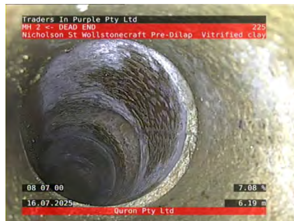
2, 00:01:23, 6.19 Junction open, good workmanship, height: 150mm at 10 o'clock
