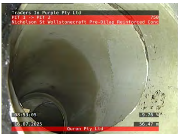
11, 00:10:18, 56.47 Connection, good workmanship, connection appears to be open, height: 300mm at 9 o'clock
