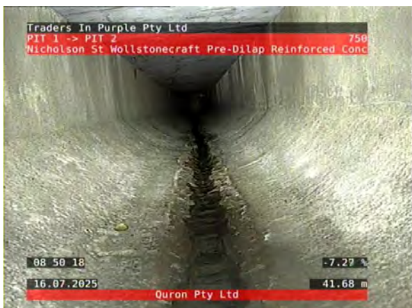
9, 00:07:59, 41.68 Longitudinal fracture, width: 2mm at 6 o'clock, Finish #
