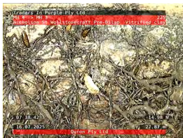
8, 00:06:28, 27.87 Fine roots--a relatively small number of flexible minor roots, at joint, Obstruction: 5-20% from 10 o'clock to 2 o'clock
