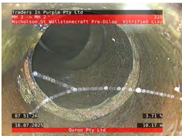
3, 00:02:36, 10.17 Junction open, good workmanship, height: 150mm at 10 o'clock
