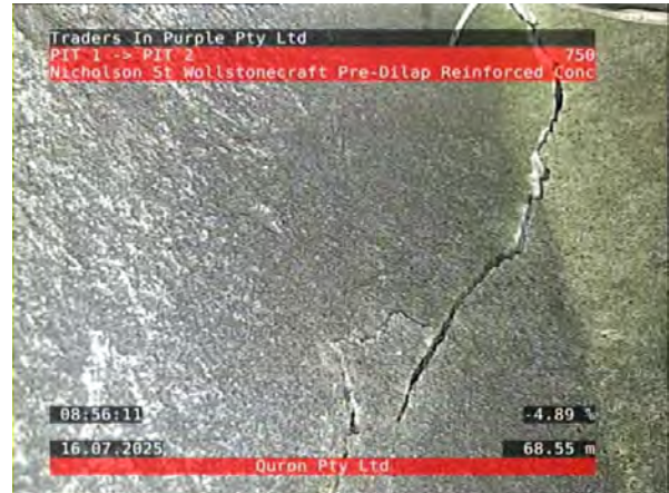
14, 00:12:16, 68.55 Longitudinal fracture, width: 2mm at 4 o'clock
