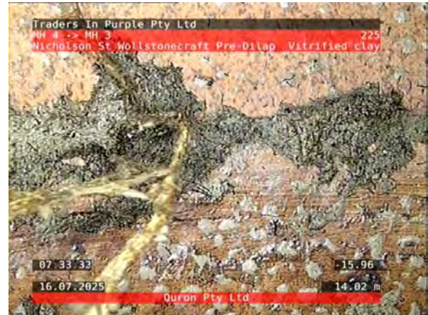
2, 00:02:44, 14.02 Fine roots--a relatively small number of flexible minor roots, Obstruction: <5% from 10 o'clock to 11 o'clock
