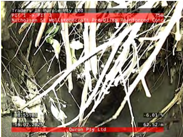
13, 00:11:24, 62.52 Obstruction, an object has been built into the structure, Obstruction: 5-20% from 10 o'clock to 2 o'clock, Start # /
