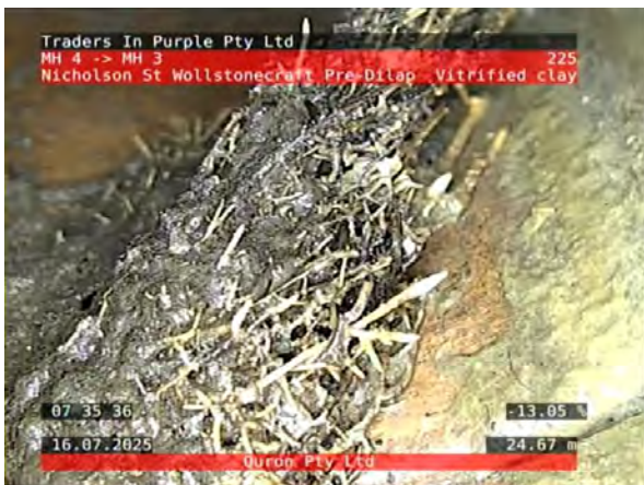
3, 00:04:38, 24.67 Fine roots--a relatively small number of flexible minor roots, at joint, Obstruction: <5% at 7 o'clock
