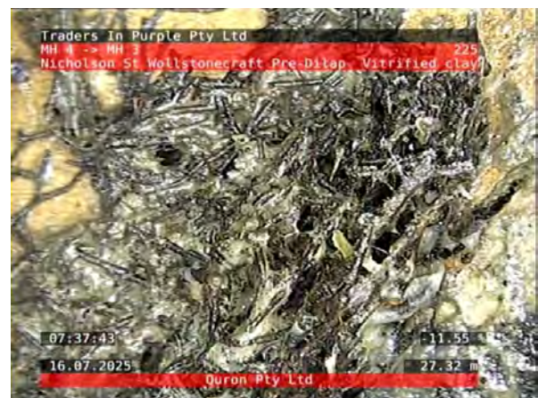
6, 00:05:56, 27.32 Fine roots--a relatively small number of flexible minor roots, at joint, Obstruction: <5% from 7 o'clock to 8 o'clock
