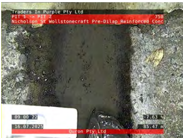
15, 00:14:38, 85.47 Other surface damage, SCOURING, Obstruction: <5%, Finish #
