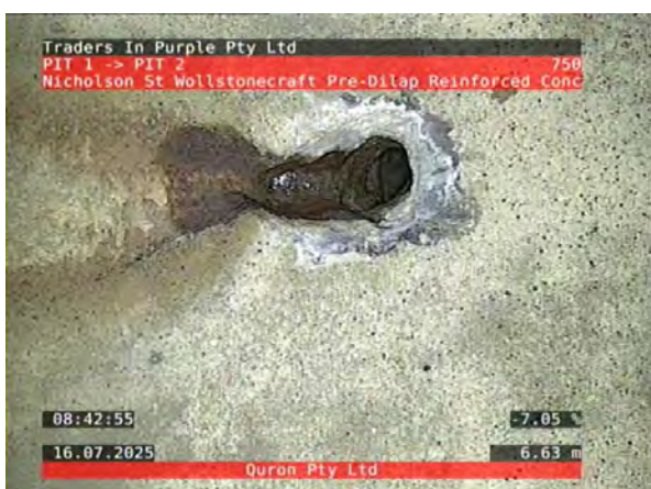
3, 00:02:20, 6.63 Hole in wall-surface damage has extended right through the wall of the conduit in places at 9 o'clock
