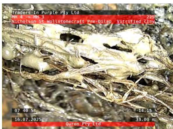
9, 00:07:52, 33.00 A mass of mostly fine roots, which has developed into an interwoven clump, at joint, Obstruction: 5-20% from 2 o'clock to
