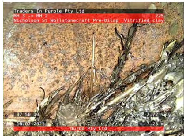
2, 00:02:00, 7.25 Fine roots--a relatively small number of flexible minor roots, at joint, Obstruction: <5% from 7 o'clock to 8 o'clock
