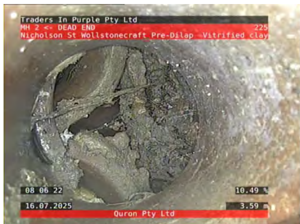
1, 00:00:50, 3.59 Defective junction, the connecting conduit is partially or completely blocked, magnitude of obstruction: >75% at 10 o'clock
