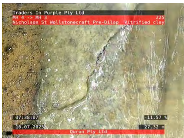
7, 00:06:02, 27.32 Circumferential wall crack, at joint, width: 0.5mm from 5 o'clock to 7 o'clock
