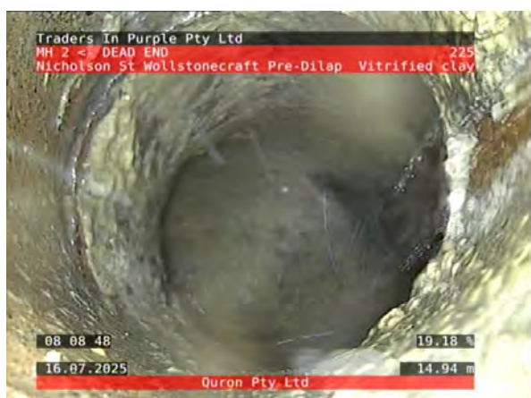
3, 00:03:03, 14.95 Junction open, good workmanship, height: 150mm at 2 o'clock
