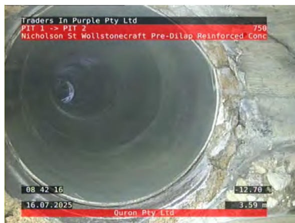
2, 00:01:46, 3.59 Connection, good workmanship, connection appears to be open, height: 150mm at 9 o'clock
