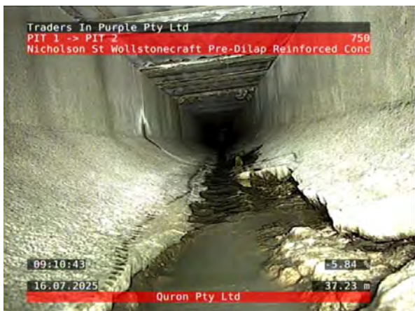
7, 00:19:05, 37.23 Breaking, some pieces are missing, length of break: 600mm from 5 o'clock to 7 o'clock / INVERT MISSING
