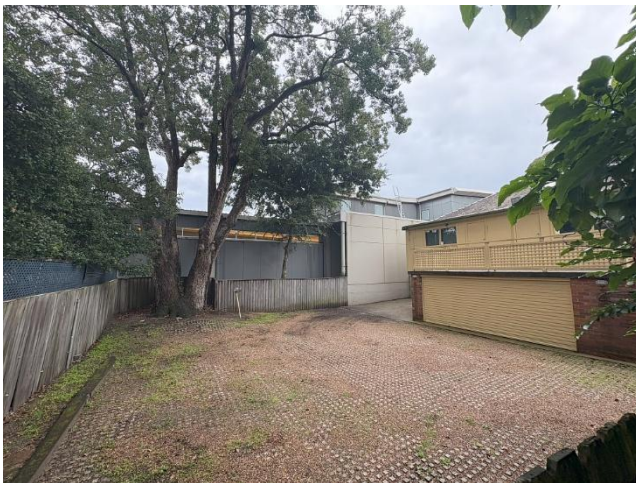
Plate 28. View north-west showing gravel-infilled cellular grid surface, tree root uplift, and partial exposure of disturbed ground in rear yard.
