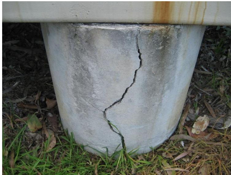
Photo 10: Cracking of the foundation casing of existing demountable buildings.
