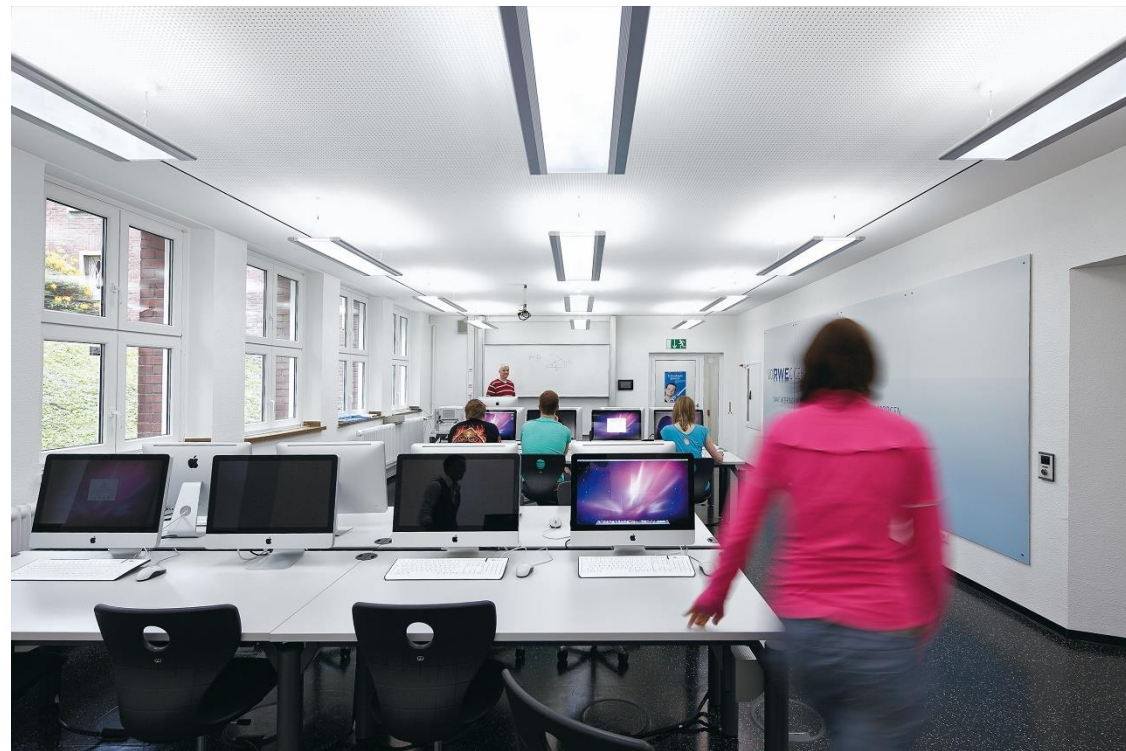
Suspended Direct / indirect luminaires within office areas
