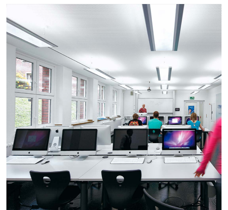
3 Suspended direct / indirect pendants to offices
