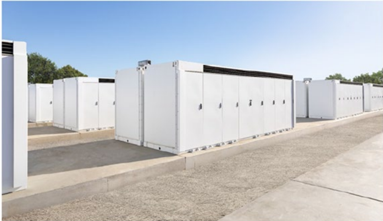
Figure 3-3: A typical BESS site
