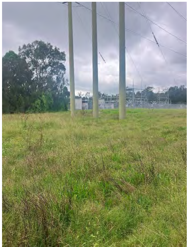
8 Looking northeast towards the Rothbury Zone Substation.
