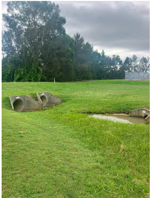
14 Drainage on the south side of the Rothbury Zone Substation.
