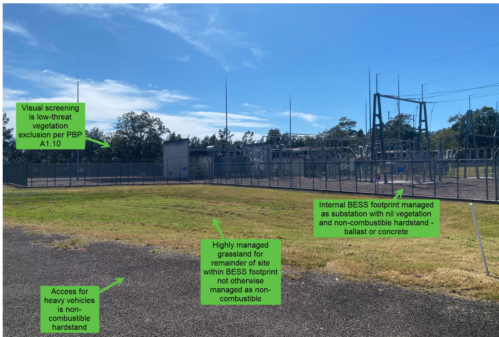
Figure 13: Landscaping management at existing Rothbury Zone Substation demonstrating BESS footprint treatment
