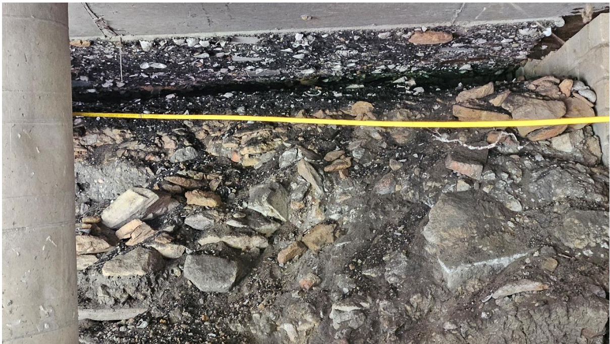
Plate 4. Dredged shell stuck to concrete from the building. (Source: Heritage Now 2024)
