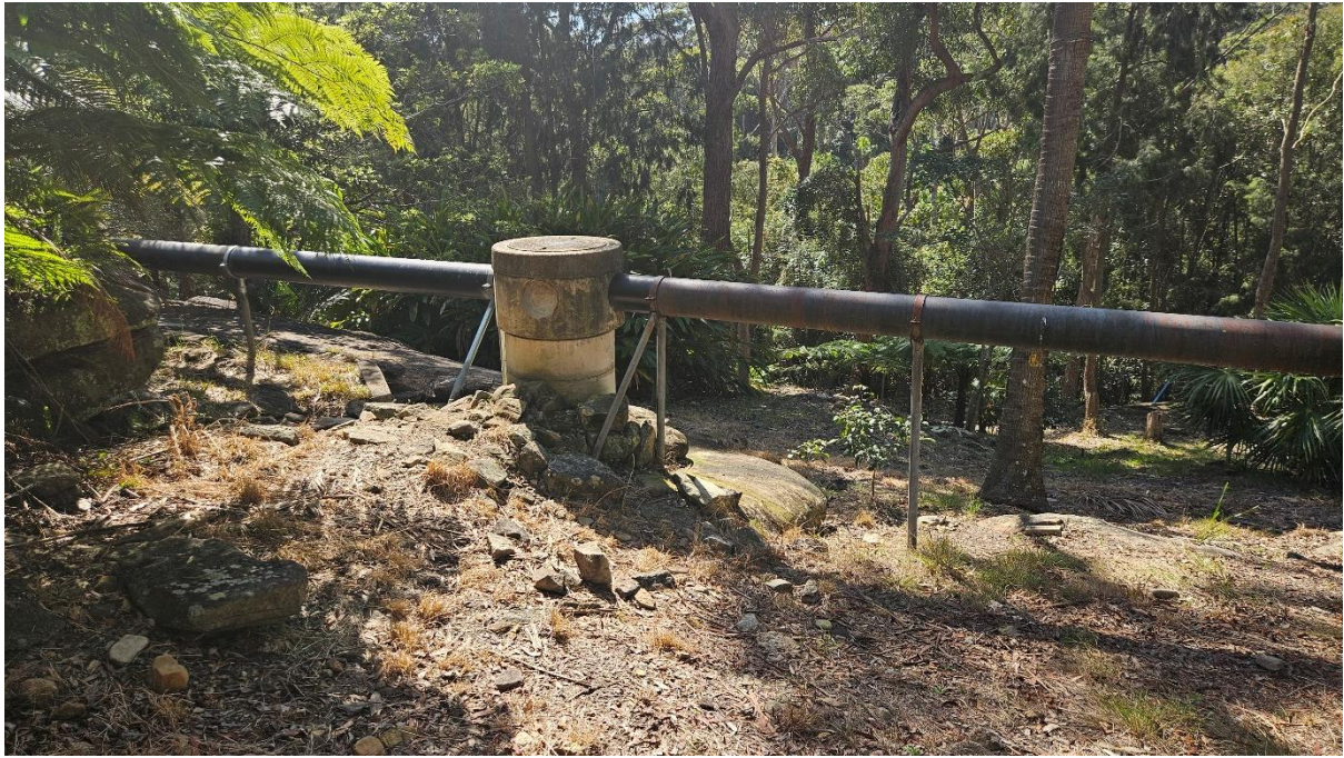
Plate 7. Above-ground water pipeline installed in a sandstone outcrop in SU1. (Source: Heritage Now 2024)
