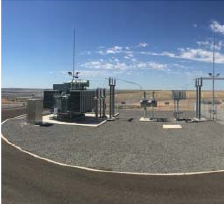
Figure 4-6 Example of a typical substation.
