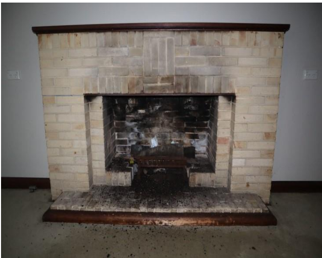
Figure 55 Living room fireplace.
