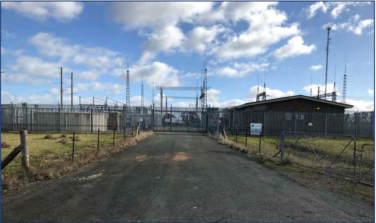
Plate 9 Finley 132 substation entrance from Canalla Road
